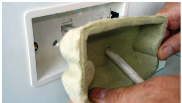
Intumescent pad being installed in a dry lining box (Photo courtesy of Knauf Drywall)
