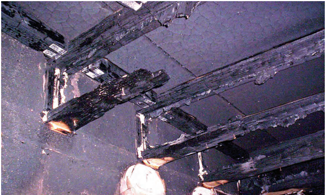
Result of an eight minute fire on lightweight joists (Courtesy of Manchester City Council - Building Control)
