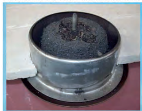
Fire Rated Ceiling Air Valve sealed after a fire
