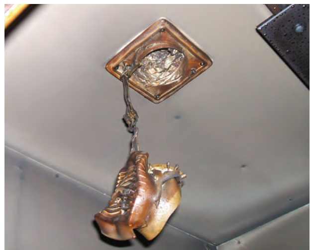
Fire spread into bathroom via plastic duct (Photo courtesy of Greater Manchester Fire & Rescue Service)
