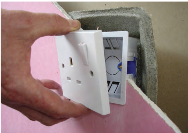
Fire and acoustic rated cover fitted behind a dry lining box (Photo courtesy of Tenmat Ltd)
