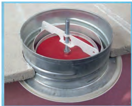
Fire Rated Ceiling Air Valve installed before a fire
